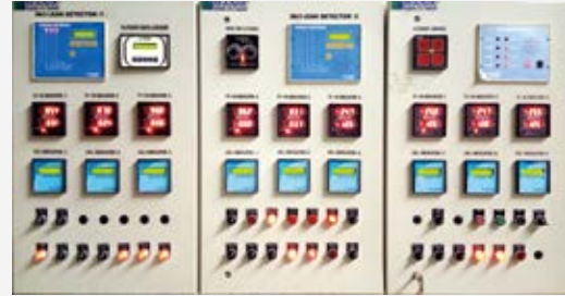
Cold Room Automation Panel
